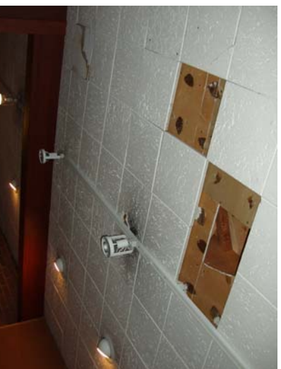
Church aisle ceilings need renovation
