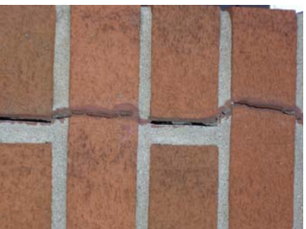
Church "steeple" is cracked
