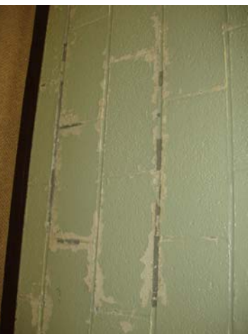
Centre needs painting
