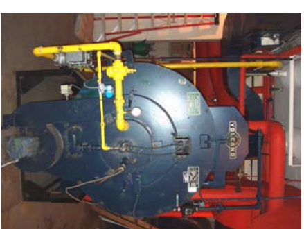
Church boiler is 50 years old!
