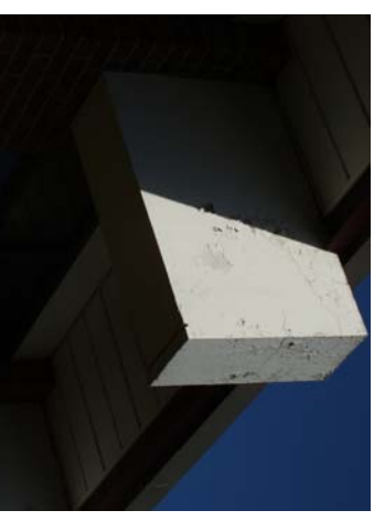
Centre concrete beams need fixing
